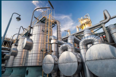
1000-E17 Heater Column
